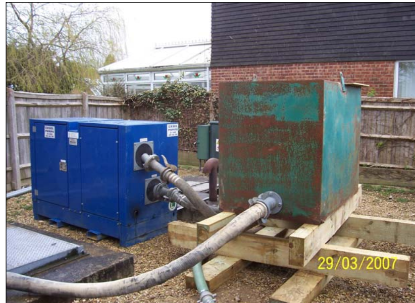
Figure A6 - Photograph of a small settlement tank usually fed by 75mm (3 inch) or 100mm (4 inch) hoses. The dimensions of the tank are 1.0m wide x 1.5m long x 1.4m high
