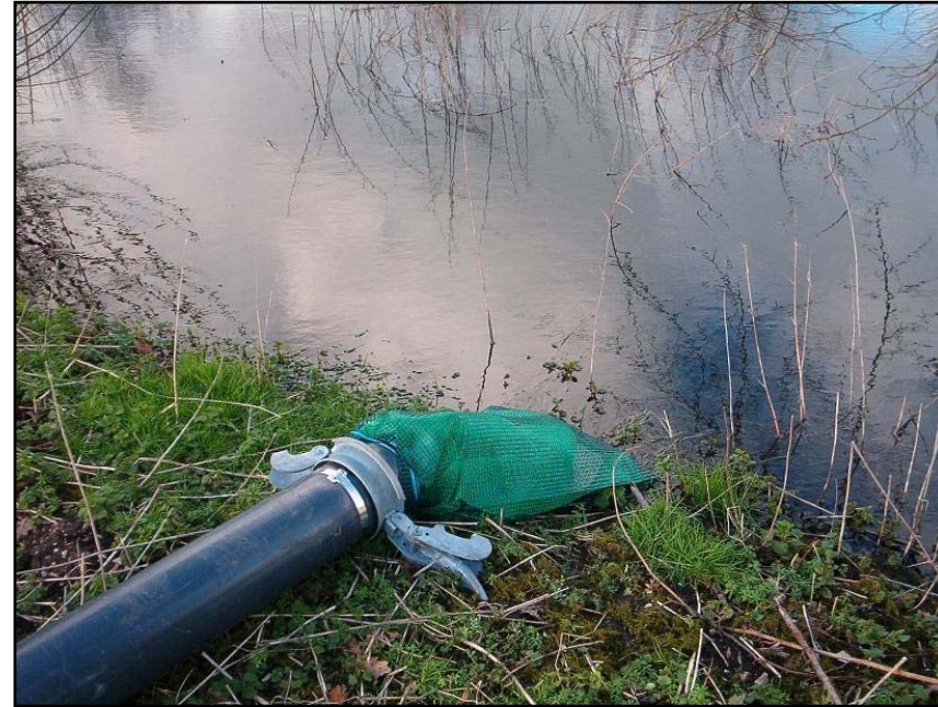
Figure A8 - Discharge of treated flow to the watercourse through a filtration sack which is replaced regularly.
