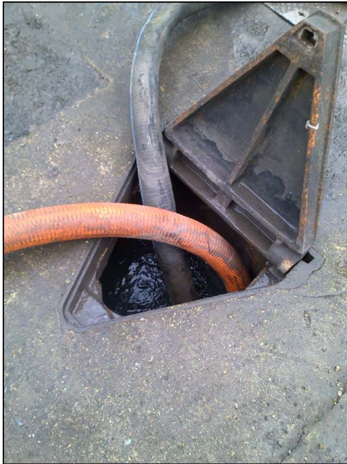
Figure A3 – Pump lifts flow through a barrel filter from a level in the sewer which captures liquid flows rather than solids
