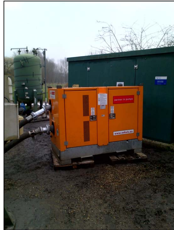
Figure A4 – Pump extracts flows from the sewer and discharges to a settlement tank
